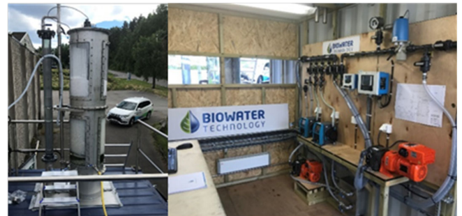
Biowater Technology HyVAB Pilot container
